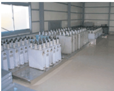
Storage of high-pressure condensers
