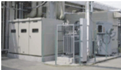
Cogeneration system at Ome Operations
