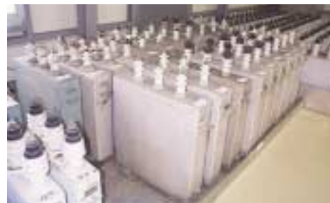
Storage of PCB-containing products on a tray
