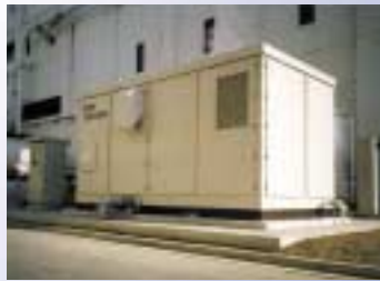
Sludge gas fuel cell power generation system
