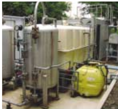
External view of a purification system
