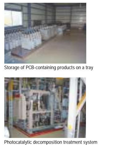
Storage of PCB-containing products on a tray Photocatalytic decomposition treatment system
